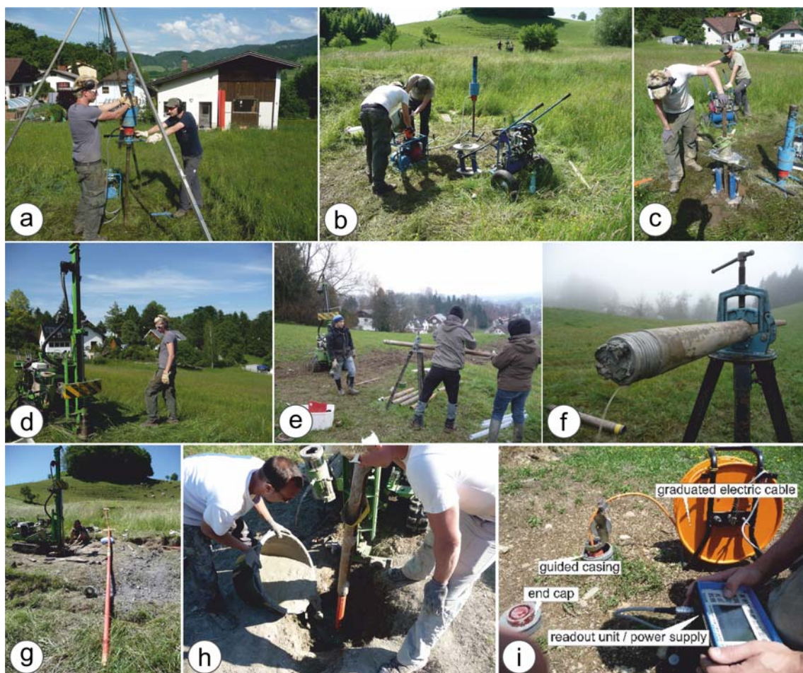
Fig. 4 Fieldwork on the Salcher landslide. a–c Dynamic probing on site DPH1. d–e Drilling operation with drill core extraction. f Water outburst of drill core B6. g–h Inclinometer installation with bentonite grout injection. i Inclinometer data acquisition (Photographs: University of Vienna (2014/ 2015))
